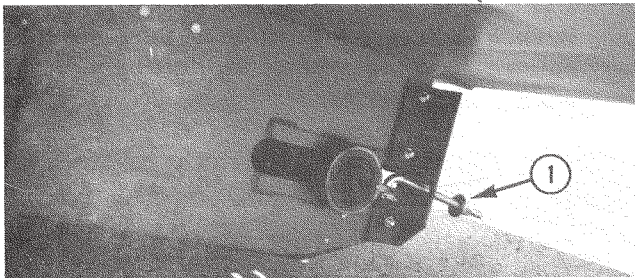
Figure 22. Conveyor Tail Pulley
